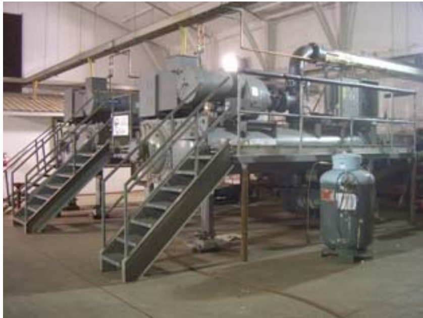
Chena Hot Springs Geothermal Power Plant Modules, installed July and December, 2006
